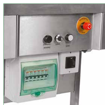
Control panel & splash proof distribution switch board
